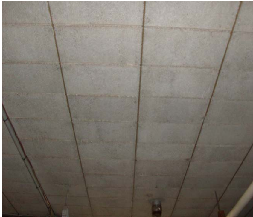
Photograph 3: View of asbestos-containing beige caulking between the gaps of the ceiling blocks in the basement (OHE sample 13462-1A).
