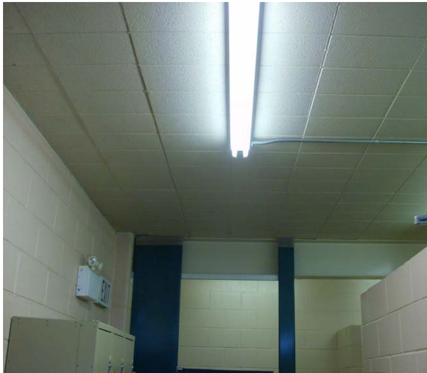
Photograph 2: View of asbestos-containing beige caulking between the gaps of the ceiling blocks on the 1 st floor (OHE sample 13216-052-1A).
