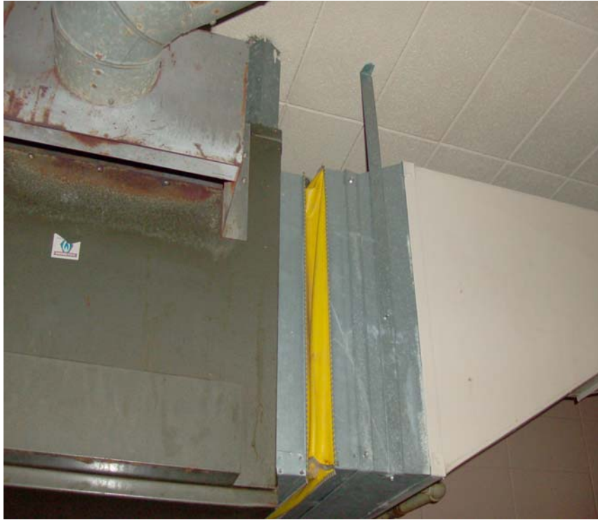
Photograph 5: View of flexible duct joint in the men's change room that could not be sampled without damaging the seals on the unit.
