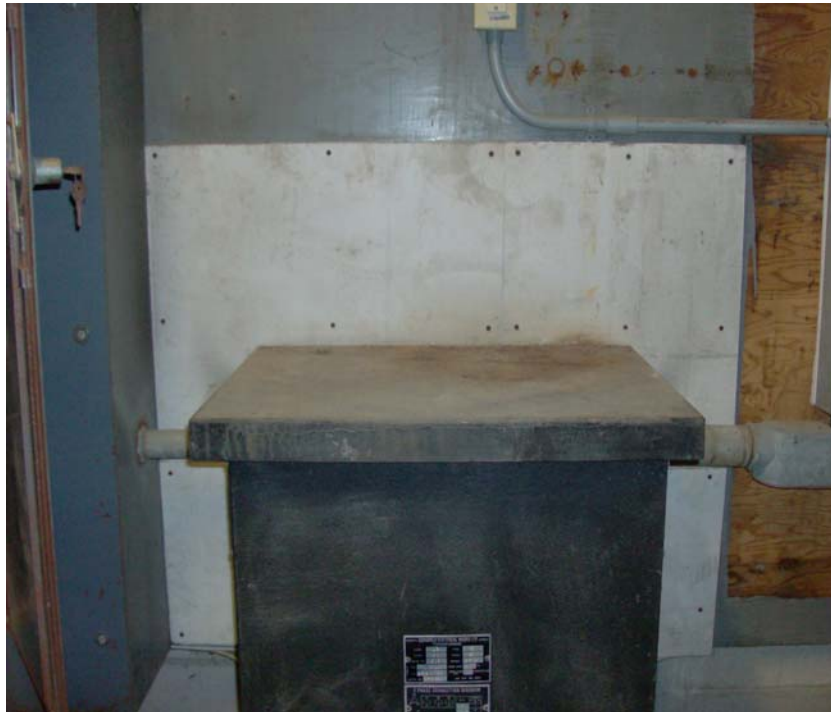
Photograph 4: View of asbestos-containing white heat shield material behind a transformer in the basement electrical room (OHE sample 13462-2A).
