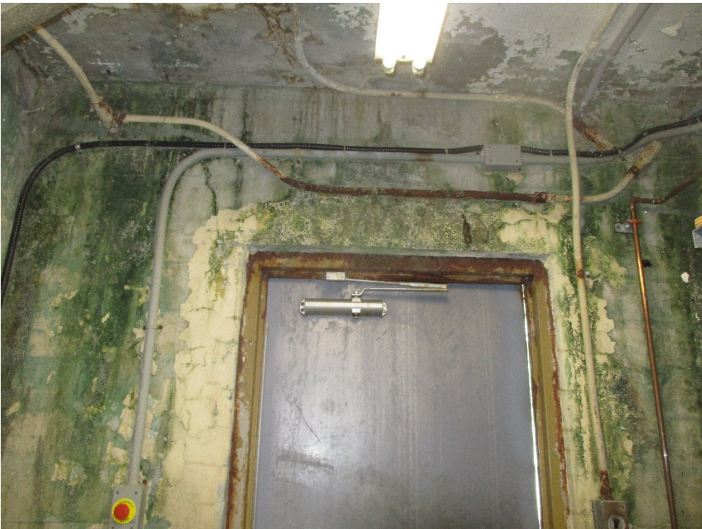
Photograph No. 4 – Laboratory analysis of discolouration on interior walls was confirmed not to be mould growth.
