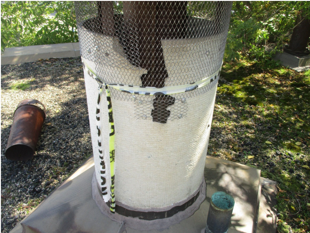
Photograph No. 2 – A transite roof ventilation pipe was observed and is deemed ACM.
