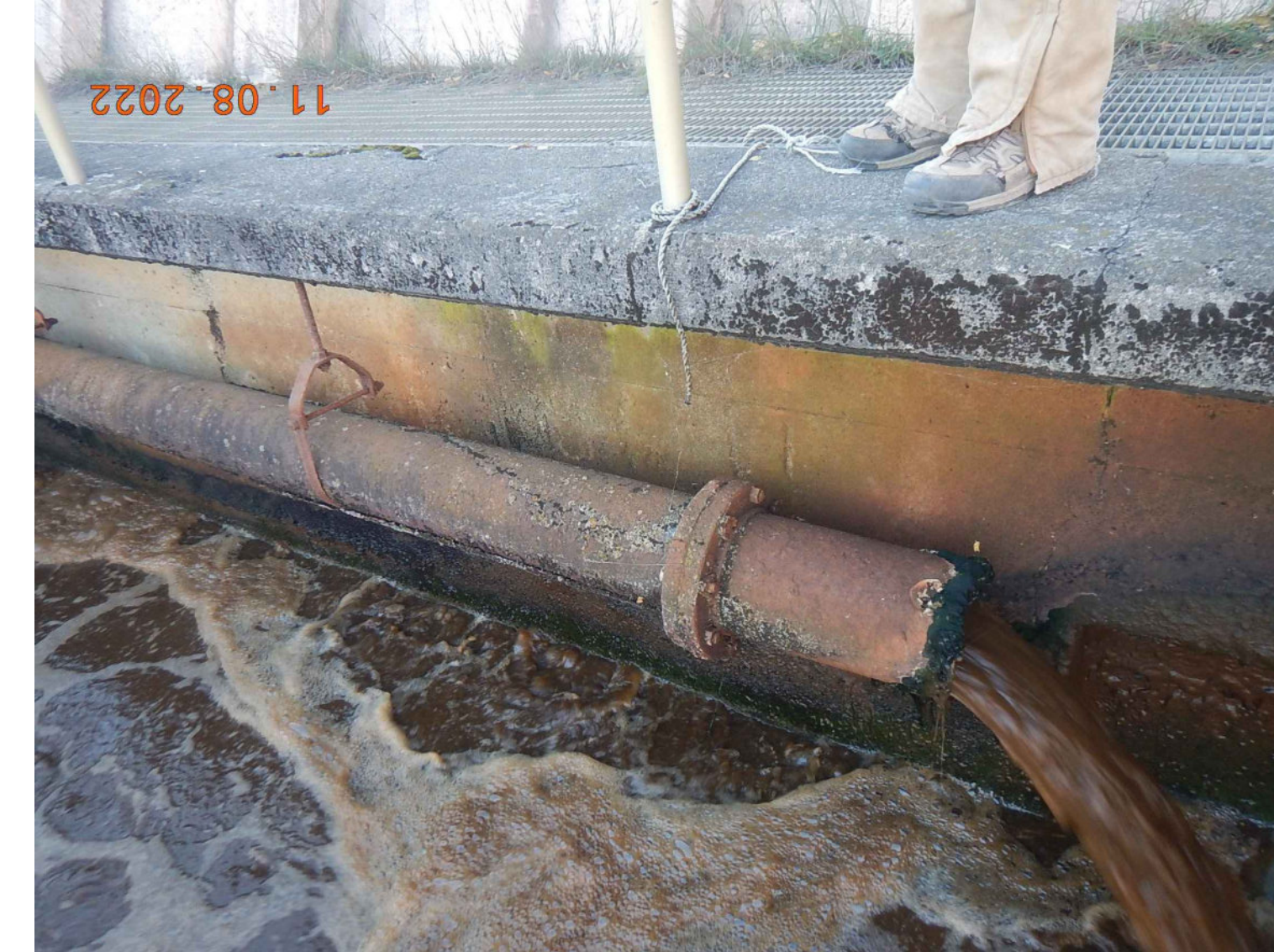
PHOTO No. 3 - EXISTING DI RAS PIPING DISCHARGE TO PLANT A AERATION TANK CELL #1 N.T.S.
