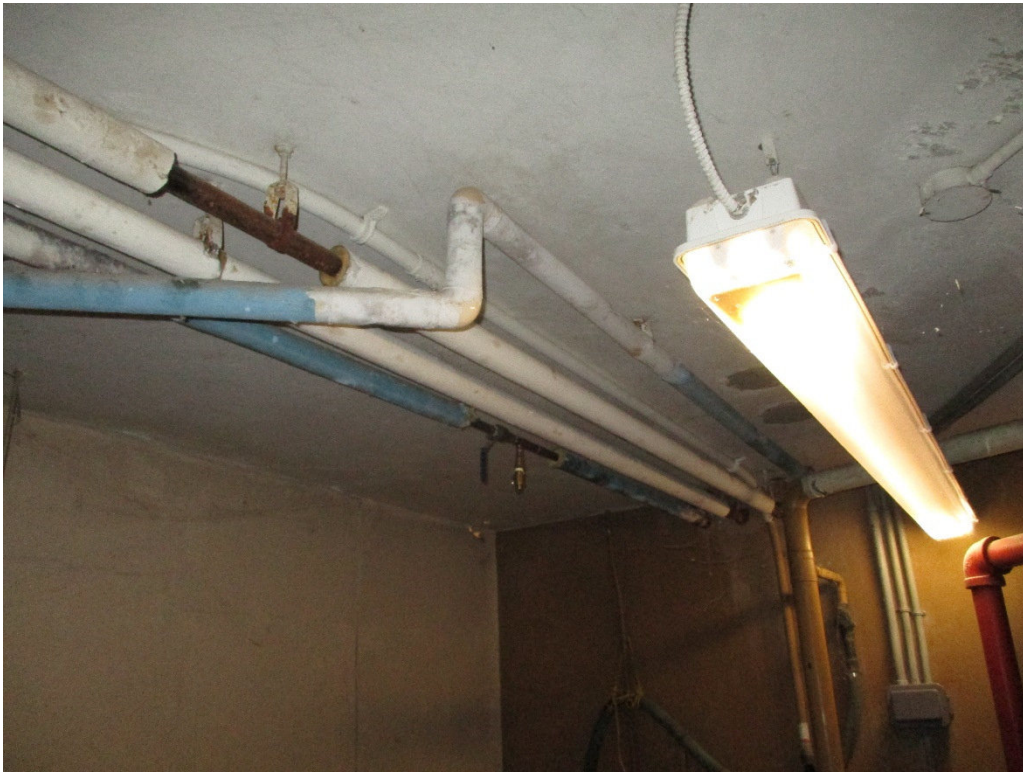
Photograph No. 7 – Fluorescent light tubes are suspected of containing mercury and fluorescent light ballasts are suspected of containing PCBs.
