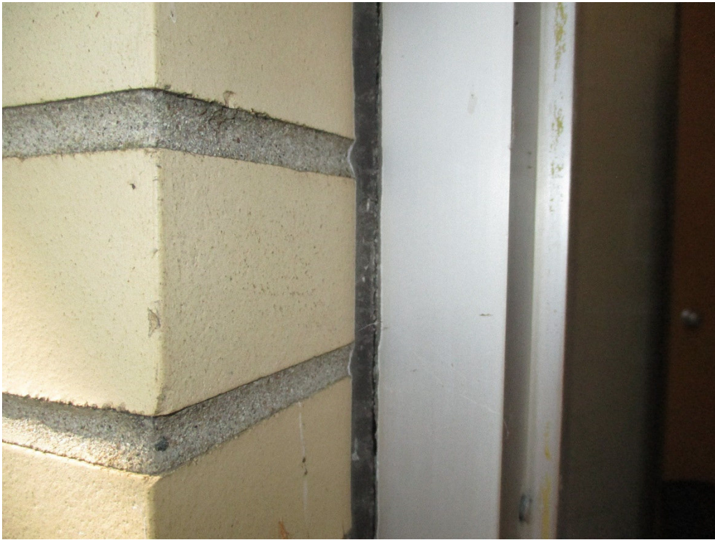
Photograph No. 1 – Exterior door sealant was confirmed to be ACM through laboratory analysis.
