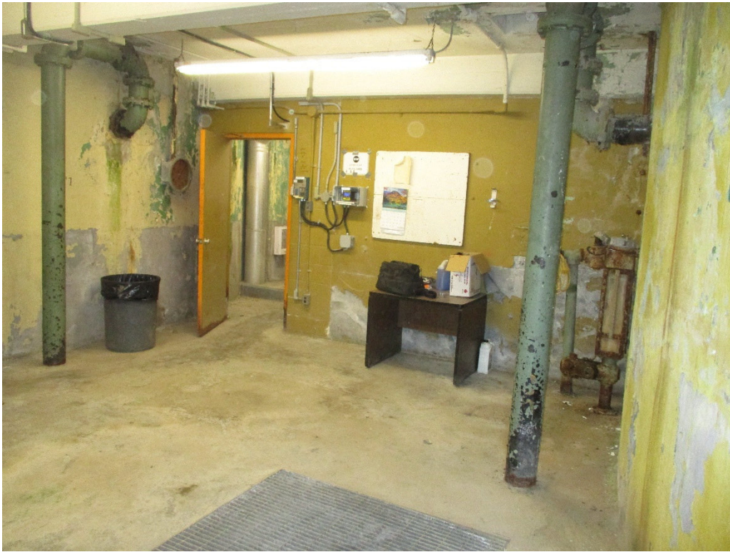
Photograph No. 5 – Lead-based, and lead-containing paints were confirmed present throughout the Site building.
