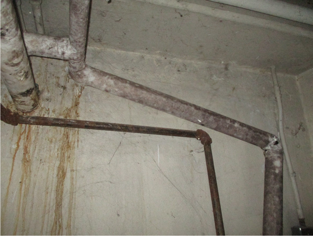
Photograph No. 3 – Laboratory analysis of discolouration on pipe wrap confirmed the presence of mould growth.
