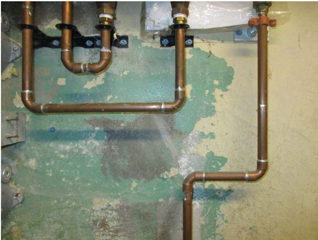
Photograph No. 6 – Solder on copper pipe joints is suspected of containing lead.
