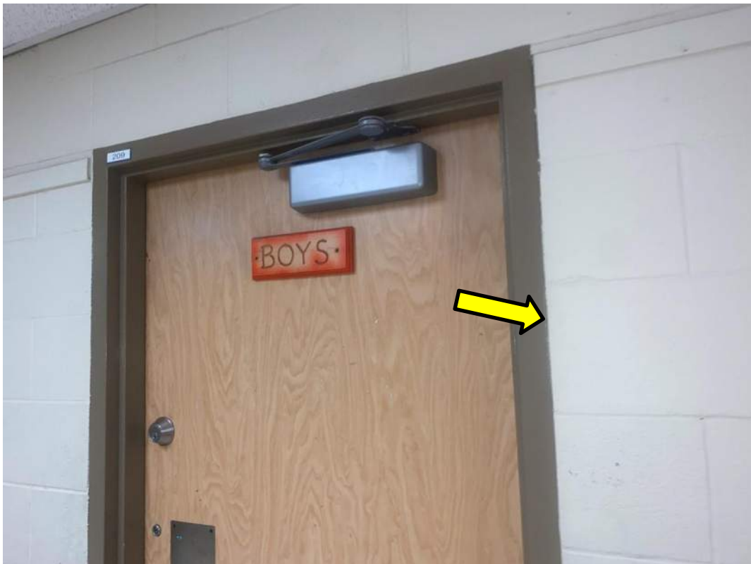
S0014A (None), white, Other, Door, Caulking, Corridor (Location #: 9264)
