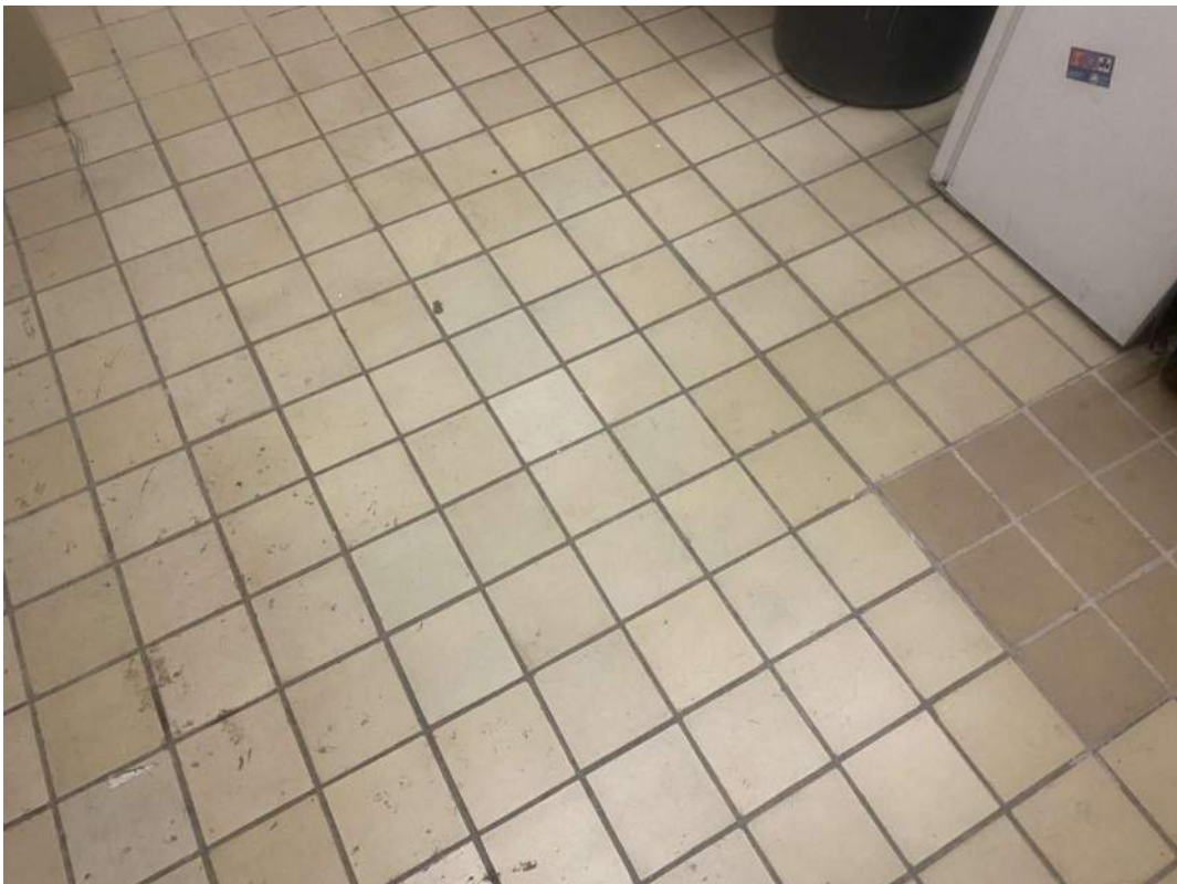
S0002A (None), Floor, Thin-set, Boy's Washroom Storage (Location #: 9213)
