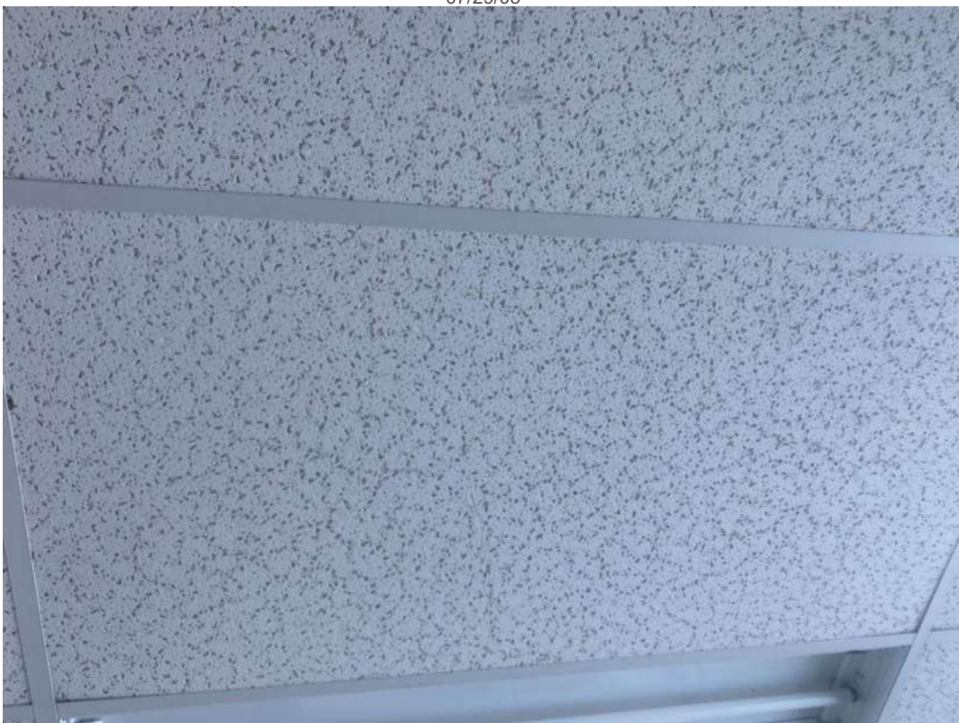
V0000 (None), 24x48 pinhole and fissure, Ceiling, ACOUSTIC TILE, Ceiling Tiles (lay-in), Staff Washroom (Location #: 9214) 08/22/11
