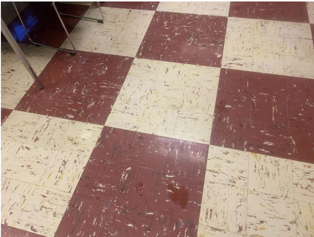
S0006A (Confirmed Asbestos), 9x9 red and yellow, Floor, Vinyl Floor Tile and Mastic, Staff Room (Location #: 9206)
