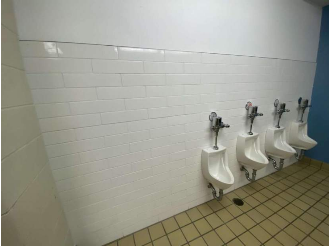
S0007C (None), Wall, Thin-set, Boy's Washroom (Location #: 9255)
