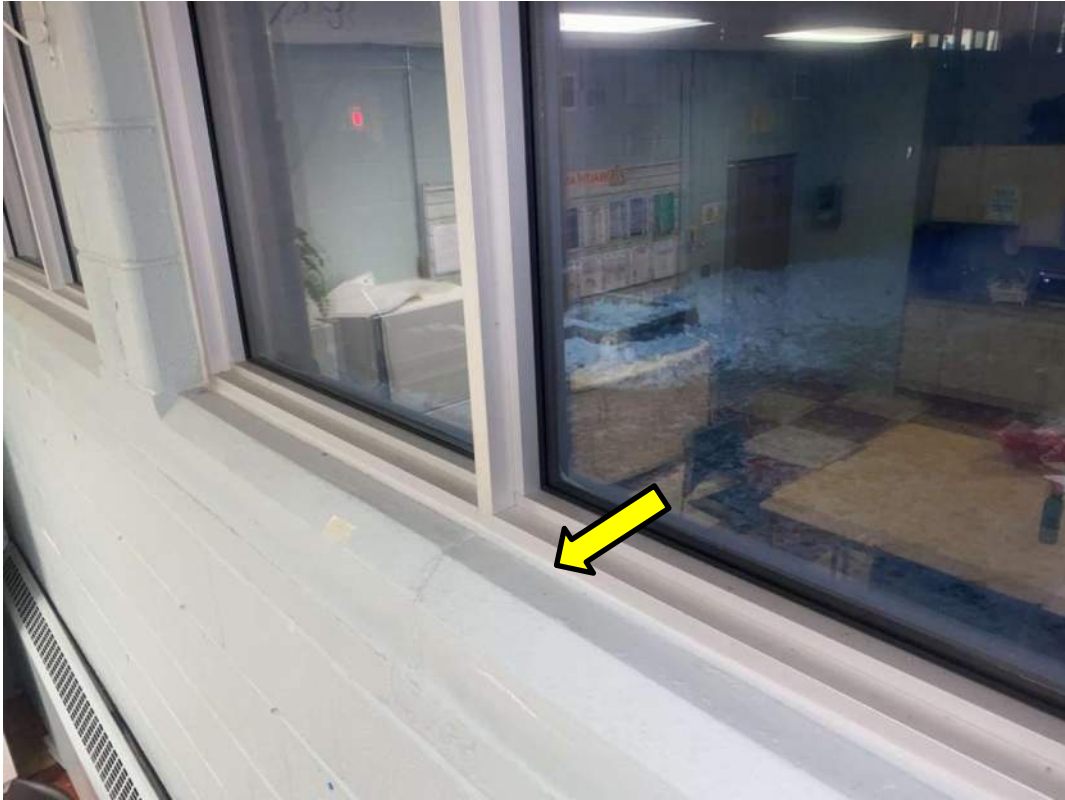
S0013A (None), light grey, Other, Window, Caulking, Staff Room (Location #: 9206)
