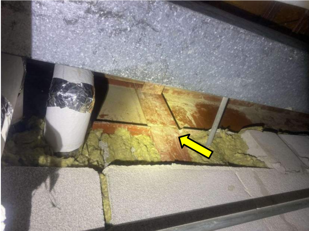
V9500(Presumed Lead), red on structural steel, Structure, Corridor (Location #: 9264)
