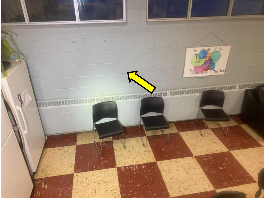
S0001C (Confirmed Asbestos), On block, Wall, Paint, Staff Room (Location #: 9206)
