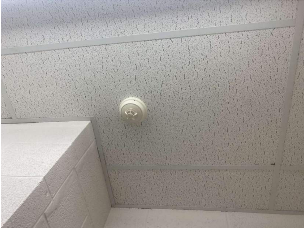
V0000 (None), 24x48 pinhole and fissure, Ceiling, ACOUSTIC TILE, Ceiling Tiles (lay-in), Male Staff Washroom (Location #: 9208) 07/29/05
