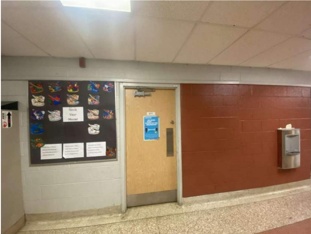
S0019A (None), outside girl's washroom door, Wall, Paint, Corridor (Location #: 9224)
