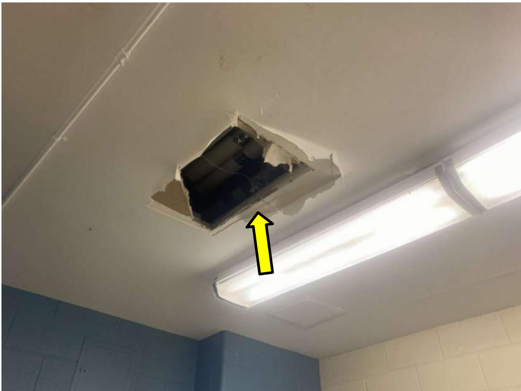
Water damage, (Presumed), Ceiling, Drywall and joint compound, Girl's Washroom (Location #: 9163)
