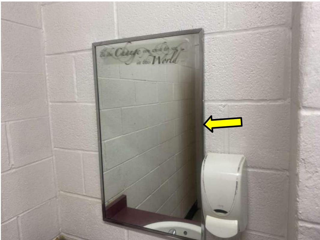
V9500 (Presumed Asbestos), Other, Mirror, Mastic, Female Staff Washroom (Location #: 9209)
