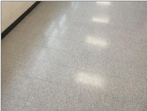
Non-asbestos 12"x12" vinyl floor tile, with asbestos-containing mastic S0059A-C, Hallway (Loc. 2029)
