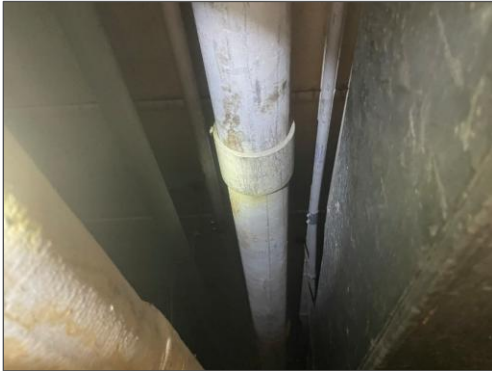
Presumed asbestos-containing transite pipe, Hallway (Loc. 1011)
