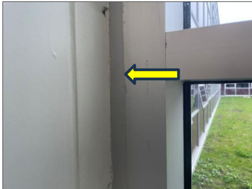
Non-PCB grey caulking, Hallway (Loc. 1011)
