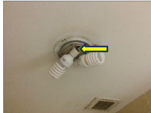
Asbestos-containing heat shield, Storage (Loc. 2045)
