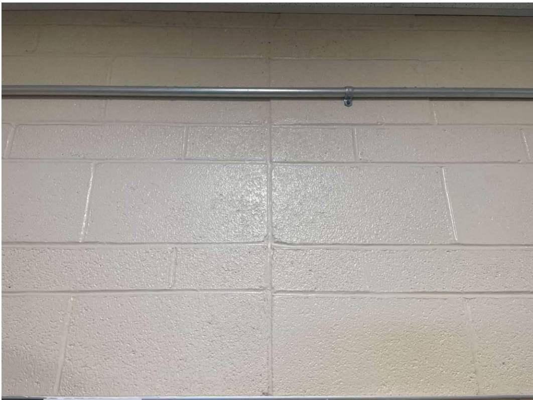
S0026A (Confirmed Asbestos), Other, Expansion Joint, Caulking, Corridor 2 (Location #: 3003)
