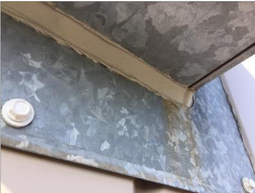
S0002A-C (Confirmed Asbestos ), Other, Caulking, Roof / Exterior (Location #: 0) (Photo from previous report)
