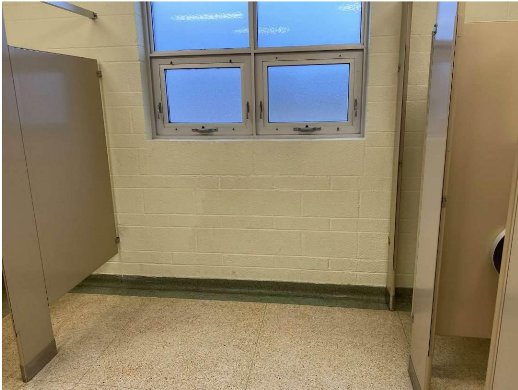
V0001(Lead, Low), Off white paint on masonry wall, Wall, Girls Washroom 2 (Location #: 2976)
