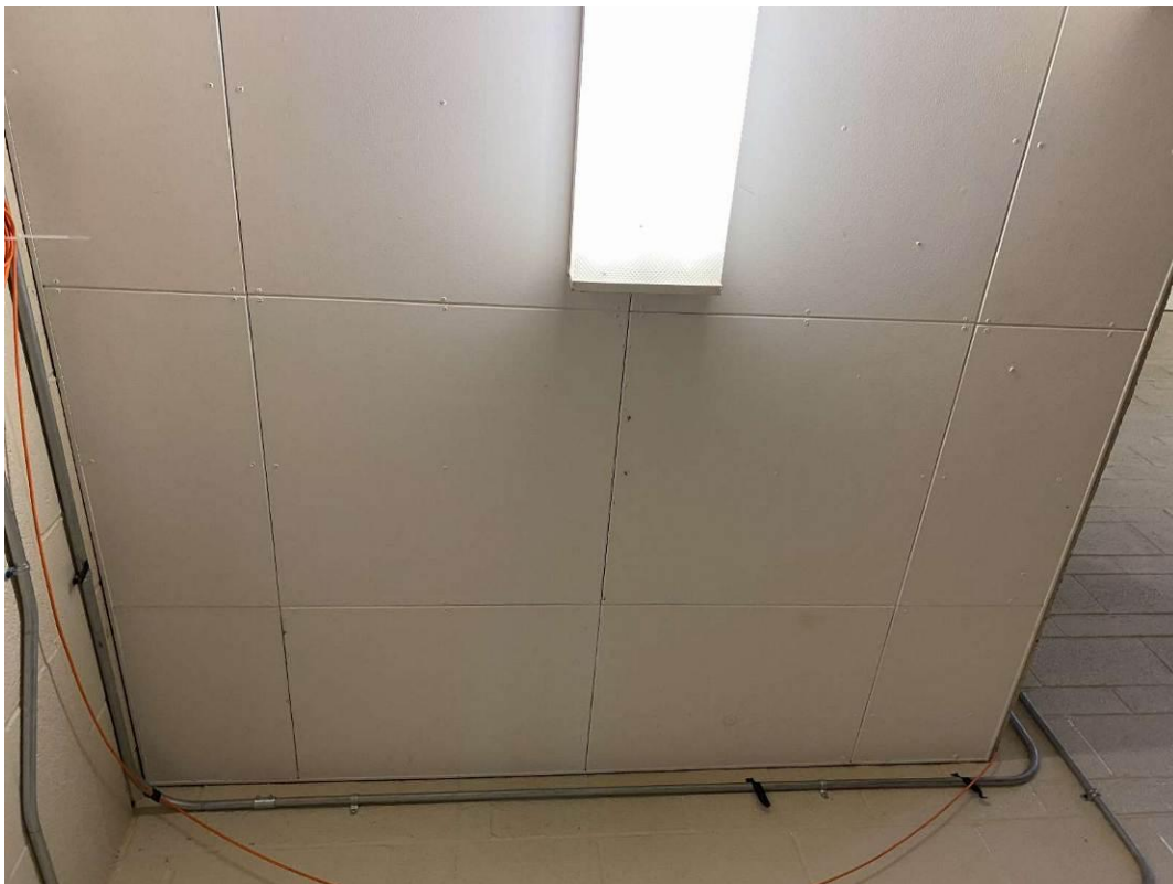
V0036 (Confirmed Asbestos), Ceiling, Cement Product (Transite), Stairwell (Location #: 2990)
