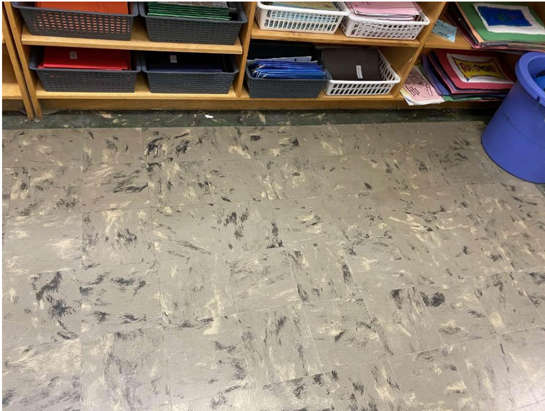
S0015 (Confirmed Asbestos), 9 x 9 grey with black and beige, Floor, Vinyl Floor Tile and Mastic, Classroom (Location #: 2991)
