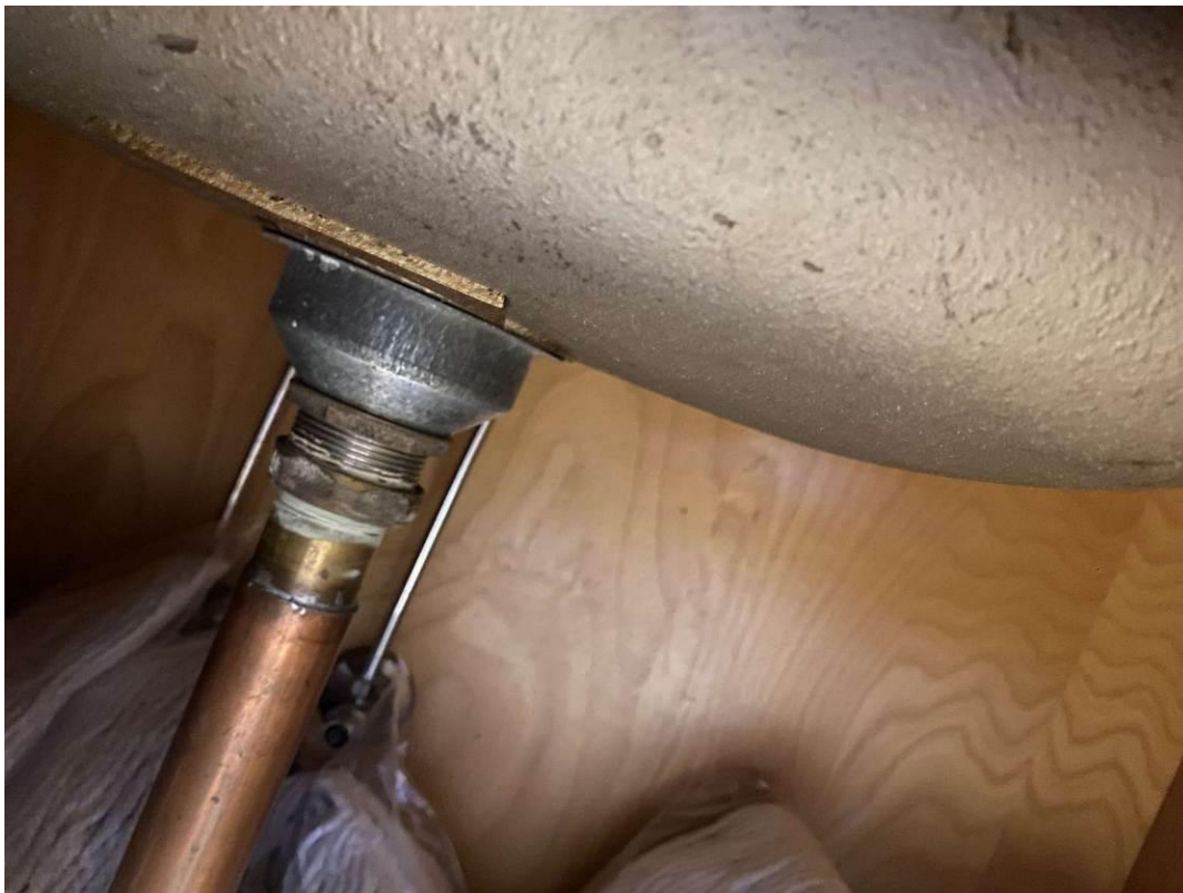
V0016 (Confirmed Asbestos), Other, Sink, Mastic, Gold, Classroom (Location #: 2995)
