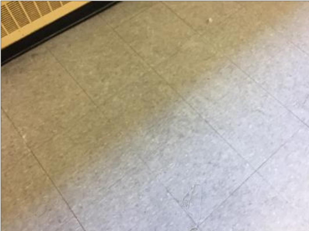
S0004A (Confirmed Asbestos), 12 x 12 grey with white fleck, Floor, All, Vinyl Floor Tile and Mastic, Learning Commons (Location #: 2972)
