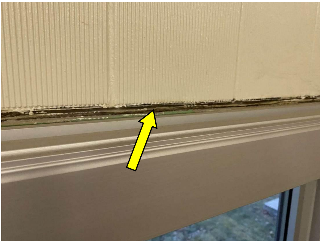
S0006A (Confirmed Asbestos), Other, Caulking, Learning Commons (Location #: 2972) White caulking on glass blocks
