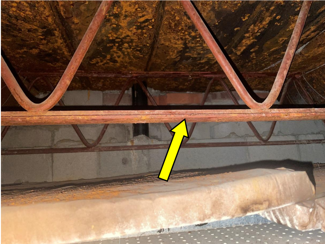
S0011(Lead, High), Red Primer, Structure, Corridor 2 (Location #: 3003)
