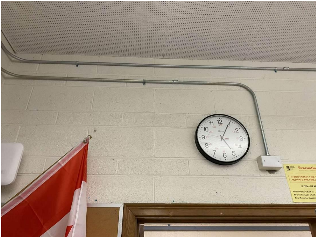
V0003(Lead, Low), Beige paint on masonry wall, Wall, Classroom (Location #: 2991)
