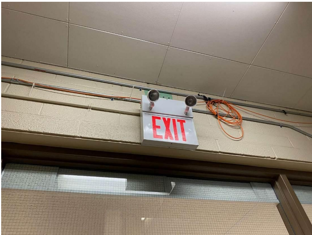
Pb Products, V9000(Yes), Batteries in Emergency lights, Stairwell (Location #: 2990)
