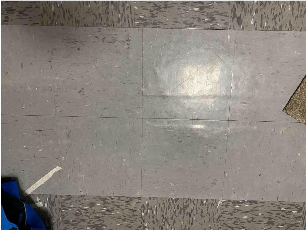
S0007A (Confirmed Asbestos), grey, Floor, Vinyl Floor Tile and Mastic, Learning Commons (Location #: 2972) Under millwork
