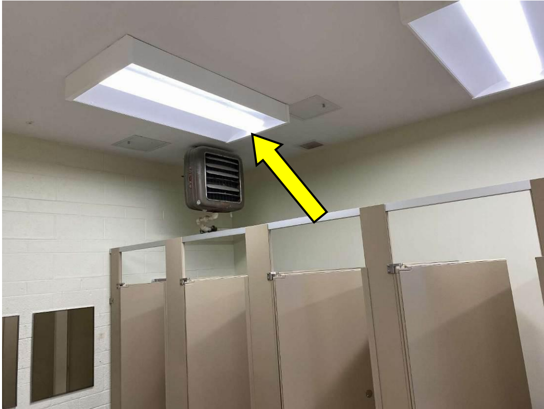
Mercury, V9500(Presumed), LIGHT FIXTURE, Girls Washroom 2 (Location #: 2976)
