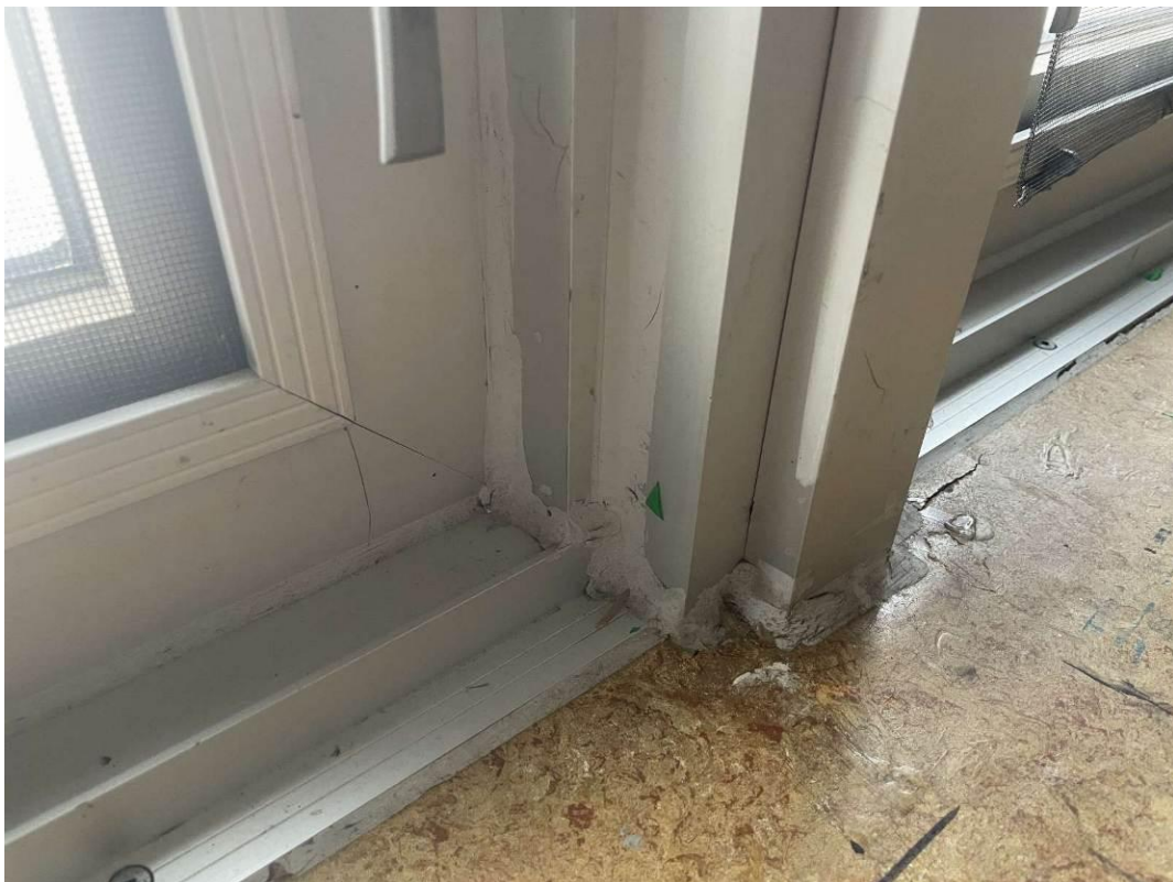
V0021 (None), Light grey caulking on windows, Other, Caulking, Classroom (Location #: 2993)
